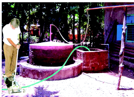
A Gobar Gas Plant
