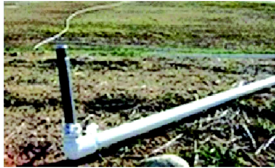
An underground sprinkler system
